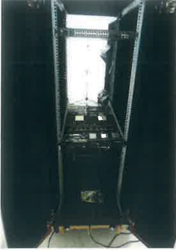
Inside of the cabinet
