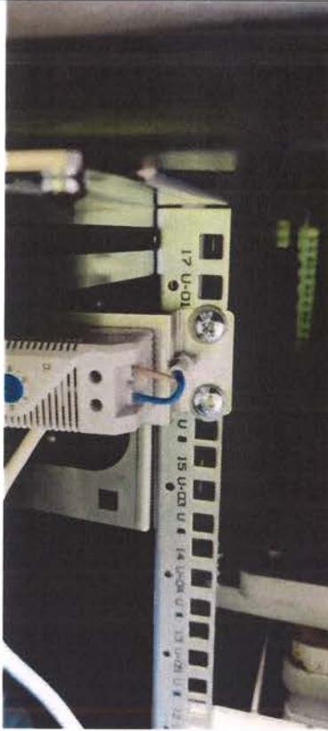
17 U (W=750X,D=1130x H=1000) Cabinet internal frame
