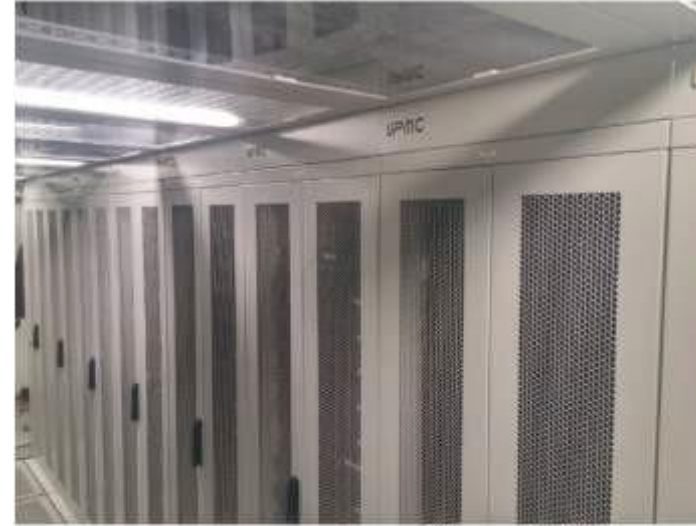
PIERRE MARIE CURIE UPMC UNIVERSITY COLD CORRIDOR APPLICATION
