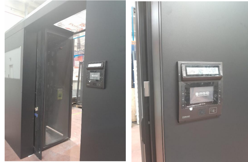
Mannai Cyber Security Ministry Cold corridor built on SE racks
