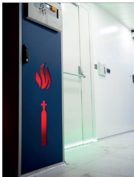
Conventional Fire Detection and Suppression System (FM200 or NOVEC)
