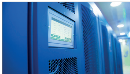
IN-Row Precision Cooling Unit
