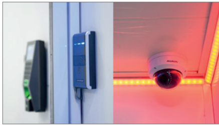
Security and Access Control
